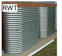
RWT RAINWATER TANKS
